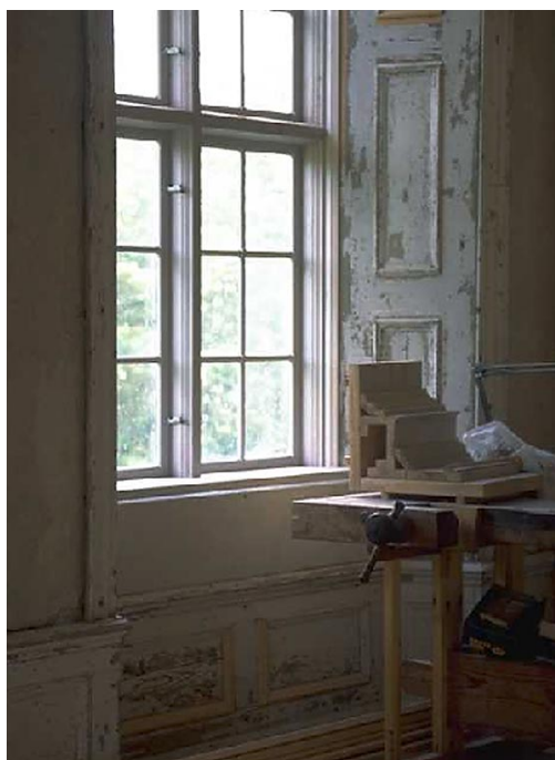
Reconstruction of 18th century windows with new cylinder glass imported from France. Mälsåker manor, Sweden. Photo Hans Sandström.
