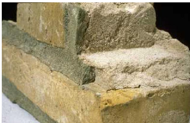
Part of a brick wall from the 1920s with lime mortar in bed and cross joints and a coloured decorative joint at the surface. Sweden. Photo Ewa Sandström Malinowski.
